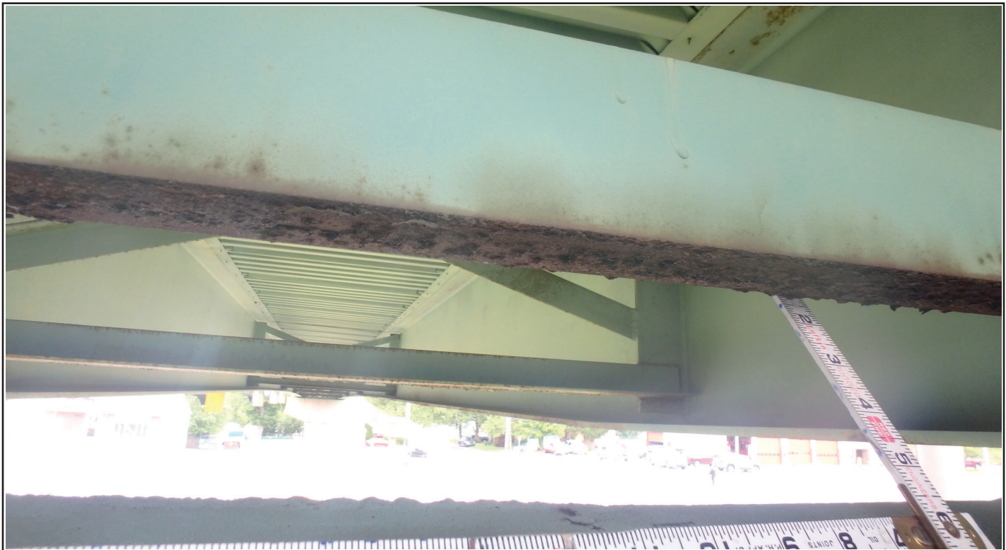
8 SP.1 DIAPH. 1 CORROSION W/LOS OVER PIER 1 FROM EAST END
