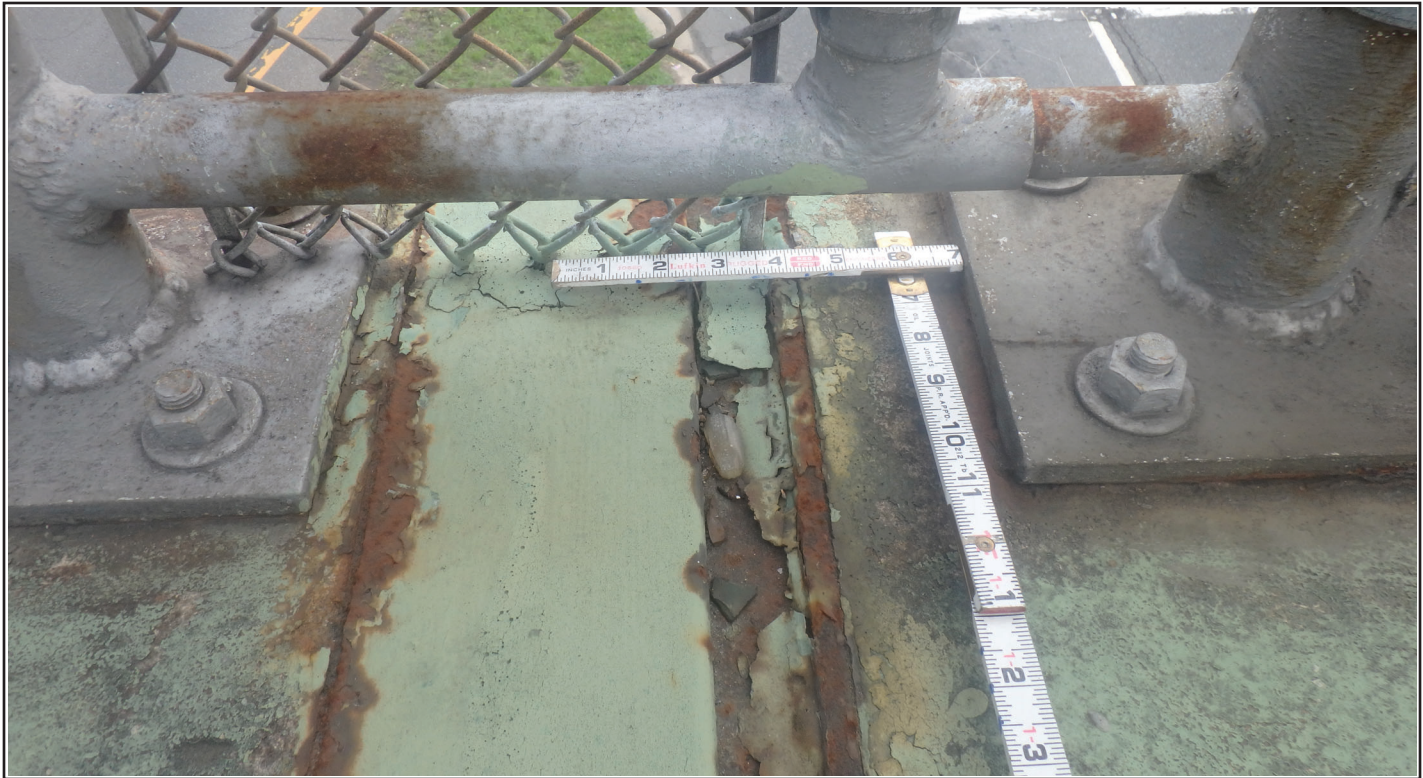
7 SP.1 OPEN EXPANSION JOINT CORROSION W/LOS AT NORTH END OVER PIER 2
