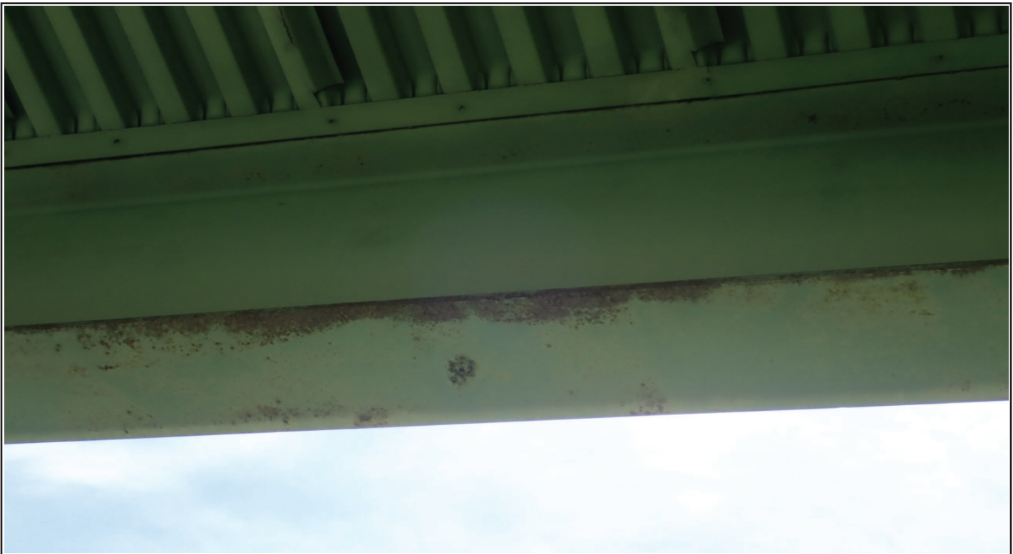
10 SP.1 BEAM 1, CORROSION W/LOS ON BOTTOM FLANGE OVER NORTH BOUND TRAVEL LANES
