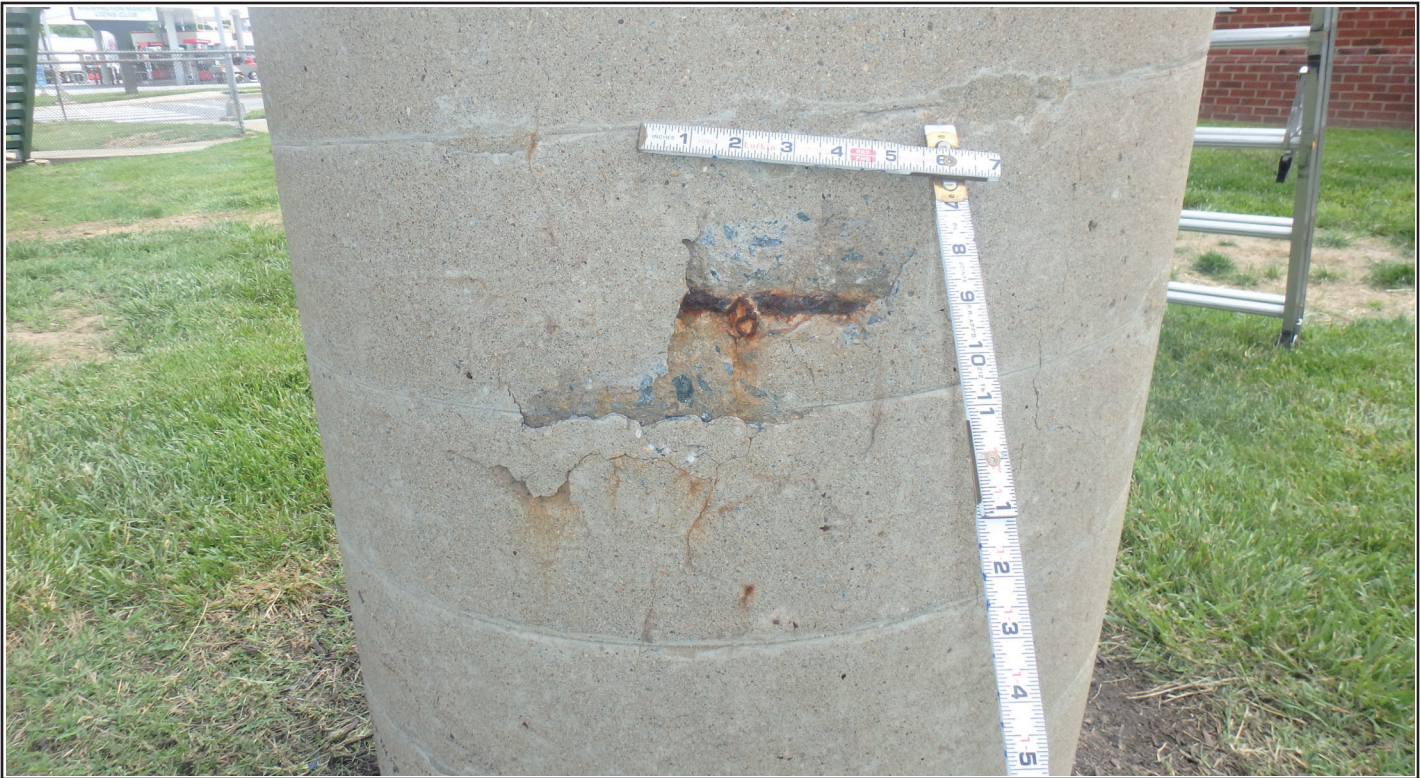
9 SP.1 COLUMN 1 EXPOSED BAR W/LOS ON WEST FACE
